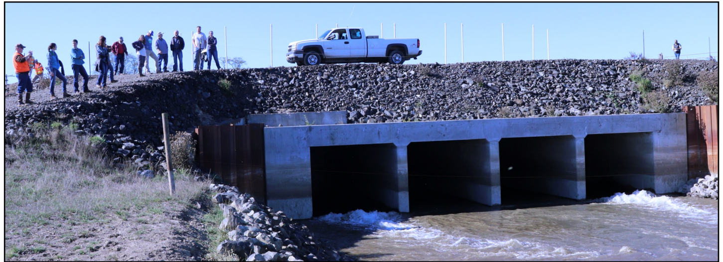
Project partners gathered Oct. 11 to see water flow through the new tide gates for the first time.
