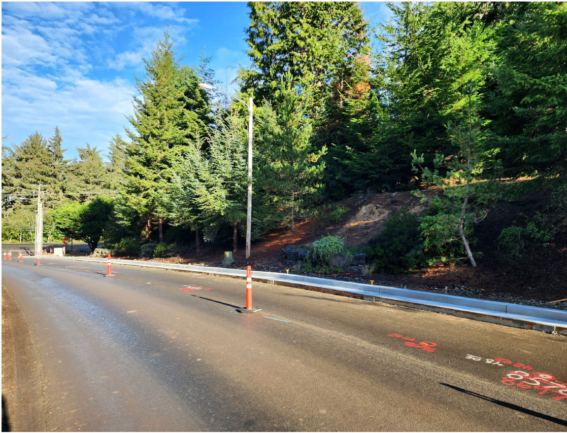
PROGRESS PHOTOS: New curbs, gutters, and formed sidewalks heading down Miluk Drive.
